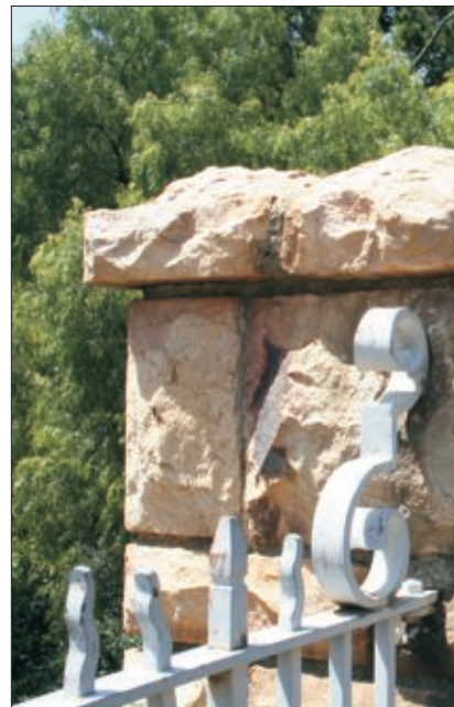
MASONRY WORK FEATURES SUPERIOR CRAFTSMANSHIP, PARTICULARLY EVIDENT FROM THE WEATHERING TECHNIQUE (THIS IS THE SHAPING OF THE UPPER COPING SURFACE TO DISPLACE WATER)
